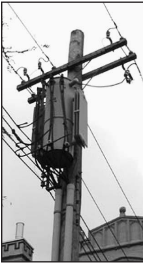
Photo #3--4kV transformer supplying secondary risers.
