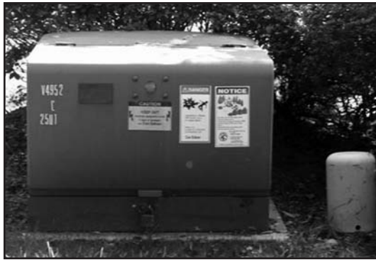
Photo #4--Pad transformer.
